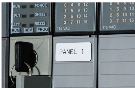
Control Panel Labels
